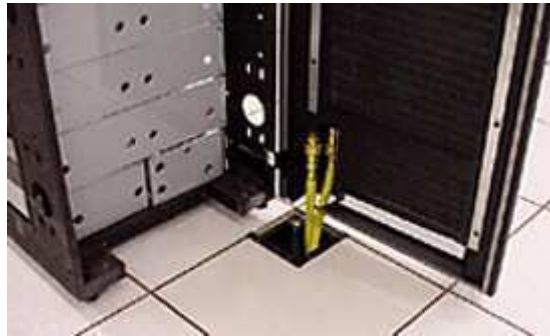
IBM's Heat eXchanger circulates chilled water from data center air-conditioning systems.
