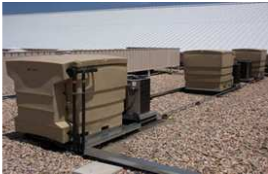
Ice Energy's Ice Bear 50 system installed atop a fitness center.
